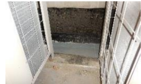
Blocked Fresh Air Intake
